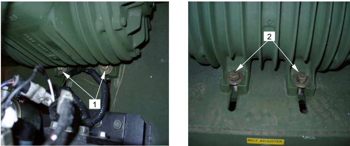
Figure 3. Tightening Vacuum Pump Mounting Bolts
