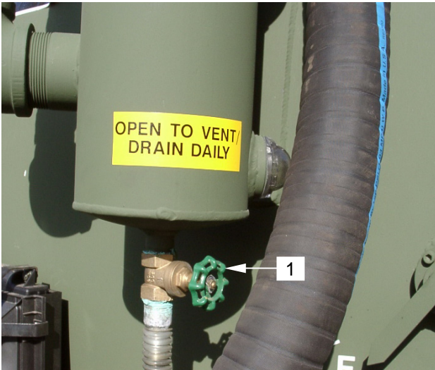
Figure 17. Moisture Trap Drain
