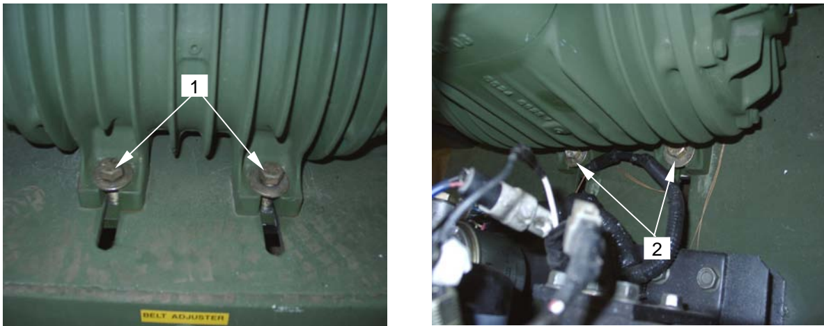
Figure 5. Tightening Vacuum Mounting Bolts
