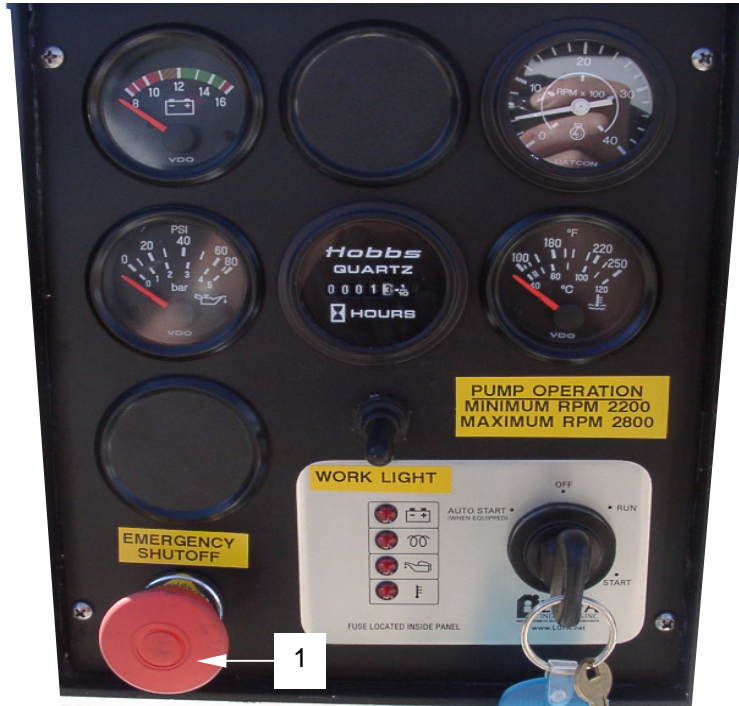
Figure 1. Emergency Shutoff Button
