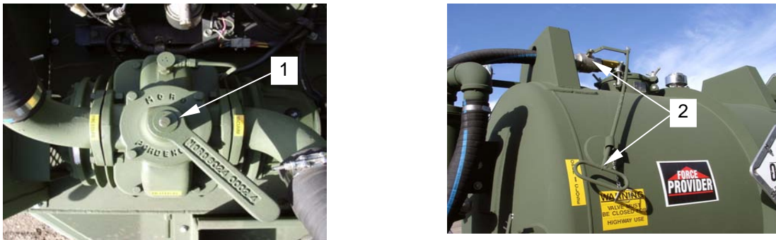
Figure 38. Pump Controls and Isolation Valve
