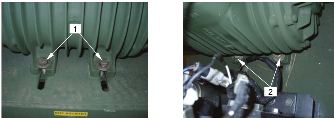
Figure 13. Tightening Vacuum Pump Mounting Bolts
